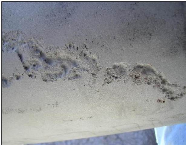
Fig. 1 – Cleaning done on this line revealed more damage than was visible during the initial inspection. Proper cleaning is essential for a good repair and excellent performance. Corrosion pitting that is visible should be filled with WrapFill 811™ .
