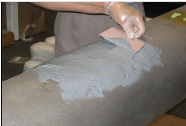
Fig. 4 – The defect must be completely filled with filler and must be flush to the surface.
