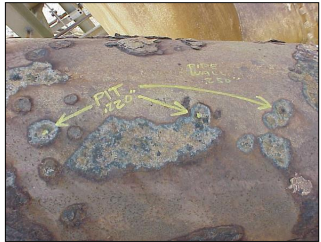
Fig. 2 – The surface preparation shown to the left is generally unacceptable . In cases where the pipe cannot be adequately cleaned, it should be noted that the final properties of the composite system may be compromised (such as inferior adhesion to the steel surface).
