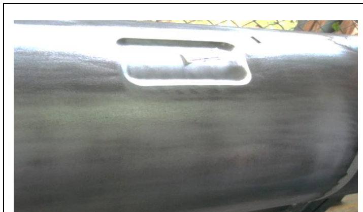
Fig. 3 – The defect must be completely filled with WrapFill 811™ repair putty and the surface must be level.
